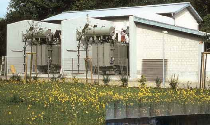
Application Public power supply system
